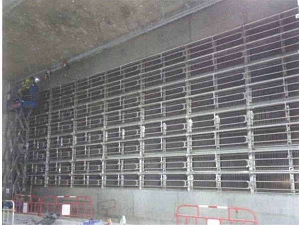
Figure 2.3: ESP Filters installed at West Ventilation Building (WVB), Central – Wanchai Bypass
